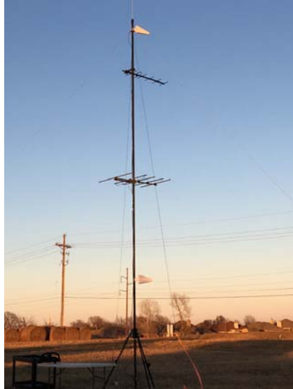
Figure 9: Base Station Mast and Antennas
