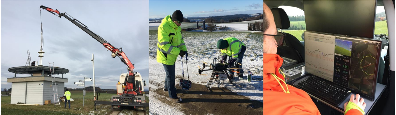
Figure 2: Emergency Replacement of Antenna System of VOR Willisau (VOR WIL). Left: Lifting of new Antenna System onto VOR; Middle: Preparation of CNS Drone by ATSEP personnel; Right: Onsite instantaneous Monitoring of Measurement Results with VOR Checker Software.
