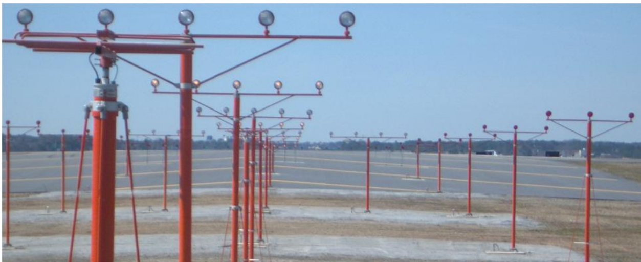
Figure 6. Example of CAT III LLZ with (Symmetrical) Approach Light Stations immediately in front of Antennas
