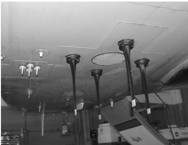
Figure 2a. DF Antenna Arrays
